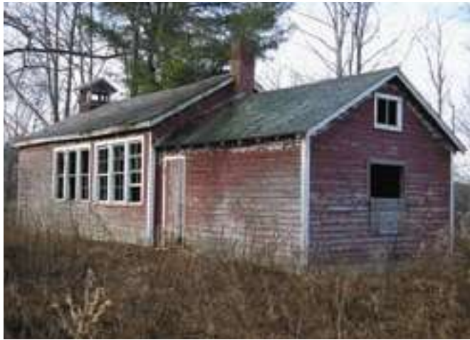
Plans call for restoring the schoolhouse so it can once more welcome children.
