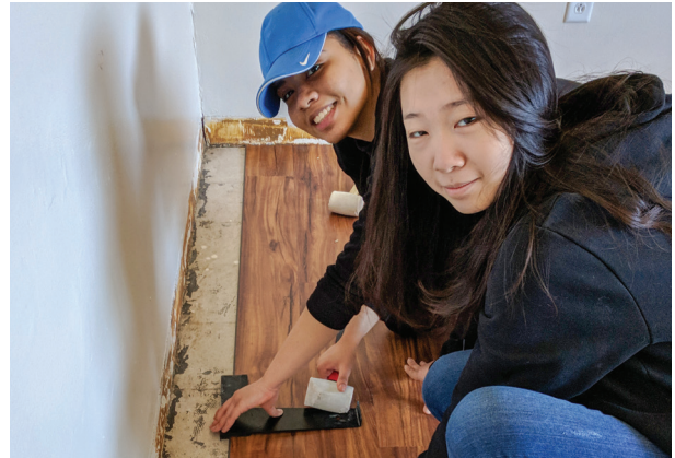
Penelope Vasquez and Wenfei Yu replace flooring in one of BMA's dorm rooms.
