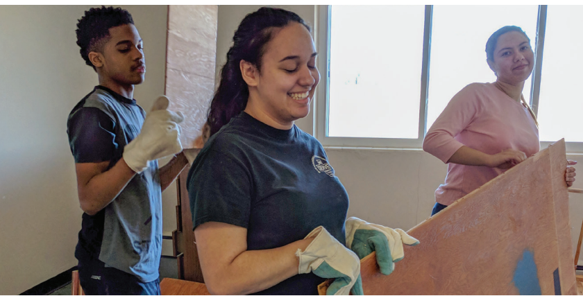
Diogenes Vargas, Maria Perez and Sofia Miquilena tear out closets and drawers during BMA's renovation process.
