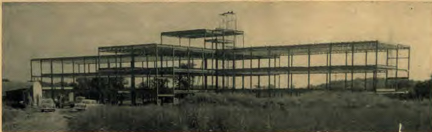
Our new hospital in Toronto takes shape. The steel framework has been completed and the masons are beginning their part of the construction. Branson Hospital will have eighty-five adult beds and a nursery of twenty-four bassinets. A nurses' course will offer the opportunity of training that Canada's young people have long wanted. The hospital will open in 1957.
