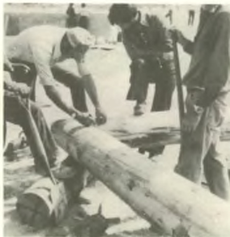
Preparing the logs which form the rustic beams for the "A" frame structure.
