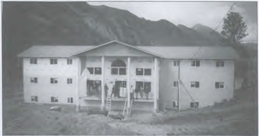
Dormitory at Fountainview Academy. Maranatha Project March 31-April 13. Both dormitories were erected in two weeks.
