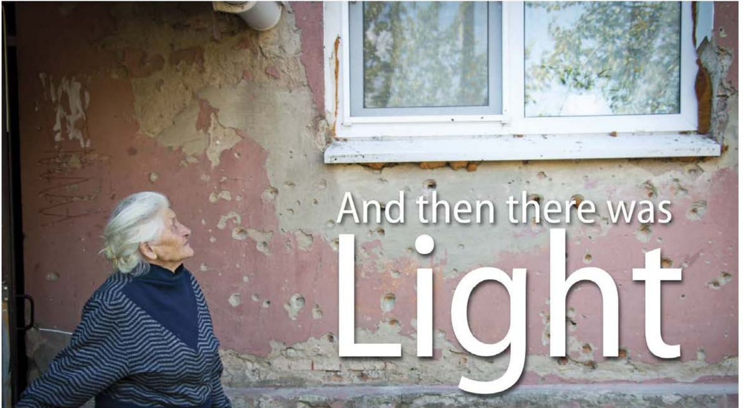
Maria views one of the new windows installed in her ground floor apartment in Schastiya, Russia. Damage from the shelling is all too apparent.
