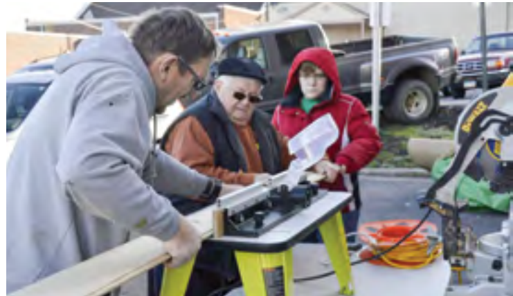
Pastor Dave Robinson enlists help from Delaware members with new paneling for the church renovations.
