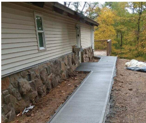
Newly completed bathhouses (which double as tornado shelters) feature exterior stonework and concrete sidewalks.
