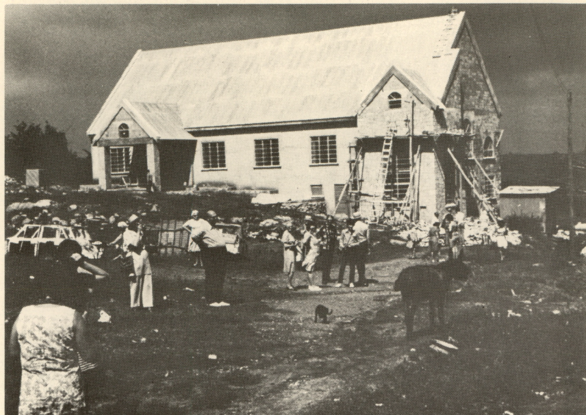
A new SDA church goes up on Antigua. It is made of native stone with an attractive green hue.
