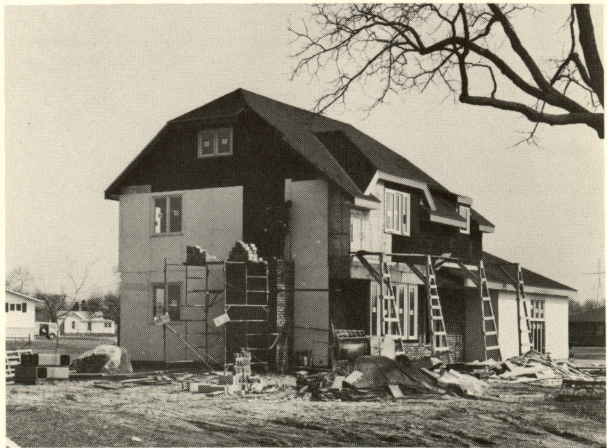
Students enrolled in carpentry, masonry, and plumbing classes of the occupational education program at Andrews are constructing a two-story English-style home on Ridge Street, Berrien Springs, for Don Gillespie, instructor in behavioral science. Electrical work in the house was done by the College class in wiring; all other work except heating and some trim will be completed by the occupational education classes. The occupational education program is aimed at persons not interested in pursuing a professional career and involves one year of classroom and on-the-job training.
