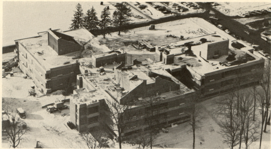
Two wings of the new science complex are well on their way to completion; the third wing is under construction. The sections housing the departments of chemistry and biology are scheduled for use this fall; the wing for physics and math is expected to be ready for occupancy by the fall of 1973. The Berrien County Drug Identification Laboratory, beginning operations soon, is being set up in the complex.
