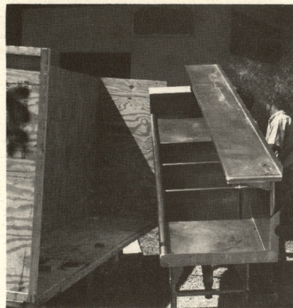
This stainless steel, 3-compartment sink is a sample of the quality of new equipment installed in the cafeteria department of Antillian College by Maranatha workers.
