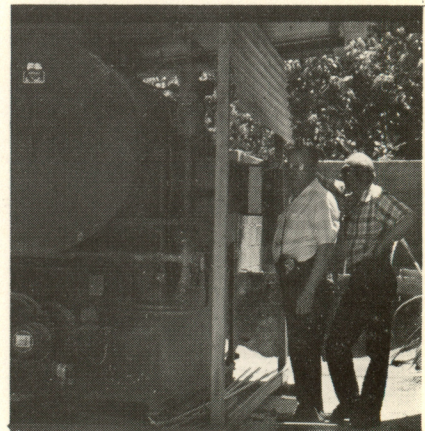
Joshua Wall, industrial education teacher at Campion (Colorado) Academy, and Lester Border, director of plant services at Walla Walla College, College Place, Washington, stand beside the new boiler they helped to install at Antillian College.
