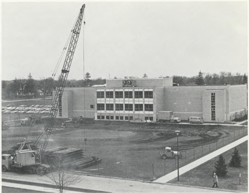
Excavation begins behind Andrews University's James White Library for an addition to the building that will double its size and triple its book capacity. The $1,250,000 construction project is expected to take 2½ years to complete. Funds for the expansion are being provided by the Seventh-day Adventist Church and various foundations, including the Kresge Foundation and the Loutit Foundation, both headquartered in Michigan.
