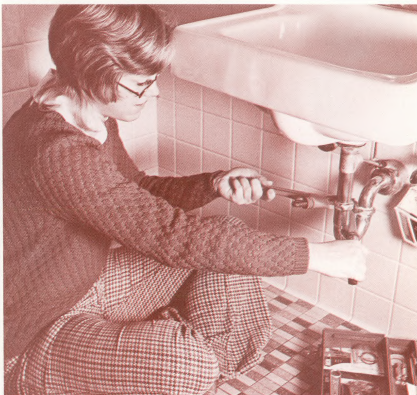
A certificated plumber from AU's Center for Occupational Education finds a job waiting in Lamson Hall.
