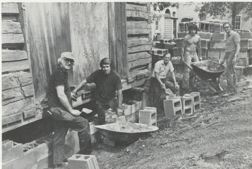
EXCAVATION, BERRIEN SPRINGS STYLE! AU personnel complete a block foundation under the old Murdock log house being restored behind the original Berrien County Courthouse at Berrien Springs. The structure is said to be the oldest two-story log cabin in Michigan and is being restored by the Berrien County Historical Commission. The log cabin was "discovered" when siding was being removed from an old building as it was being torn down. Helping from AU with the foundation are, from left, Dr. Gerald Herdman, Don Prior, Melvin Anderson, Gary Prior and Roland John.
