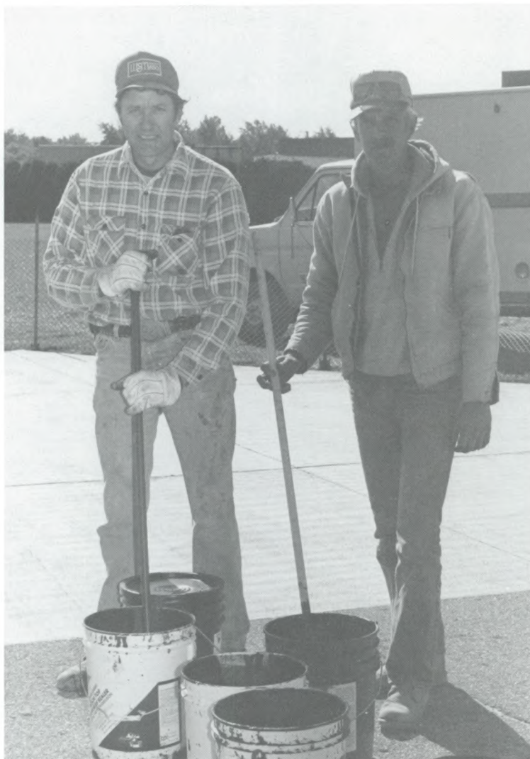
Jerry Kantor of Kantor Construction and employee Al Ziemke install a concrete slab in the RMES playground.
