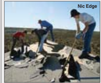
Clint Lawson, Casey Michel, Calvin Tabor and David Bryson begin removing the old roofing.
