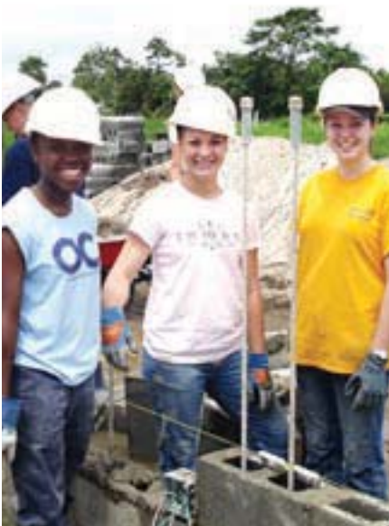
Seniors Tricia Jackson, Megan Hilde and Amanda Stevens quickly learn the art of laying bricks during their spring break mission trip in Ecuador. Classmates in the Philippines and in Kenya also participated in construction projects over spring break.
