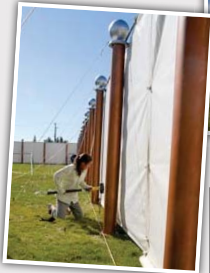
The total number of stakes pounded into the ground to set up both the tabernacle and courtyard fence is about 600.
