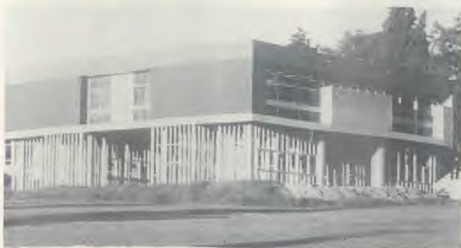
During the quinquennium many campus improvements were made. This shows the new library extension under construction.
