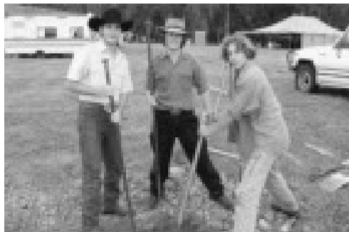
James Higgins, Juri Megaritty and George Siems of Wauchope church working on the agriculture complex's foundations.
