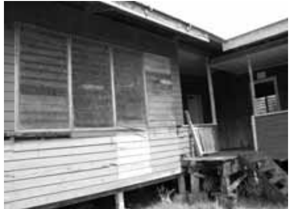
The Viru Clinic in the Solomon Islands Mission, which is desperately in need of repair.
