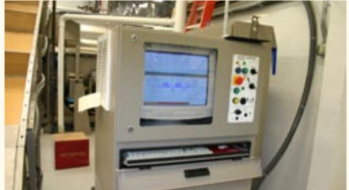
Computers control the operation of the laundry equipment.
